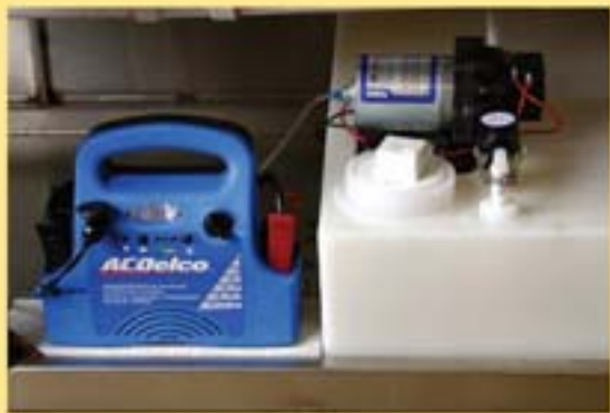
Battery pack and 12 volt pressure pump.
